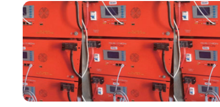
South Africa Project Telecom Power Backup 48V 200Ah
