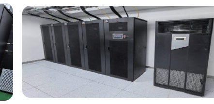
Shenzhen Project Data Centre Power Backup Project 512 V 560 Ah
