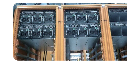
Hebei Project HVDC Power Backup Project 768 Wh
