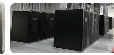
Chongqing Project Data Centre Power Backup Project 512V 280Ah
