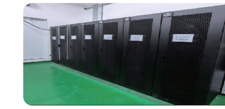
Ningbo Project Data Centre Power Backup Project 512 V 420 Ah
