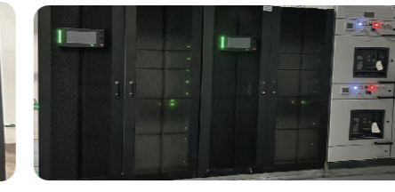
Mexico Project Data Centre Power Backup Project 512V 280Ah
