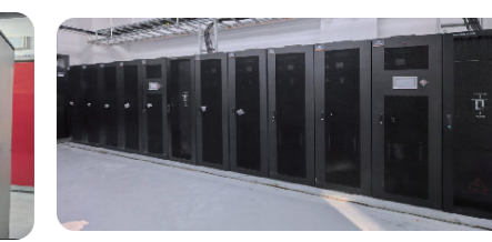
Mongolia Project Data Centre Power Backup Project 512 V 800 Ah
