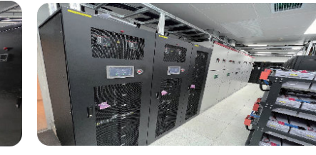
Jinan Project Data Centre Power Backup Project 512V 420Ah
