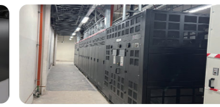
Thailand project A, TikTok Project Data Centre Power Backup Project 512V 350Ah
