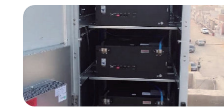
Mauritania Project Telecom Power Backup 48V 200Ah
