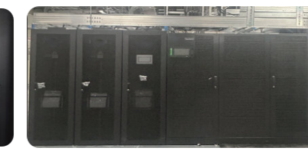
Hangzhou Project Data Centre Power Backup Project 512V 420Ah
