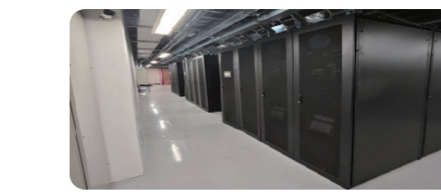
Malaysia 01, AWS Project Data Centre Power Backup Project 512V 280Ah
