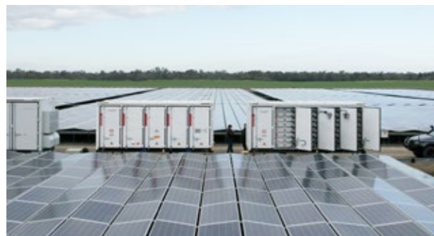
5MW/11MWh Kanowna Solar Farm Stage 2 New South Wales, Australia
