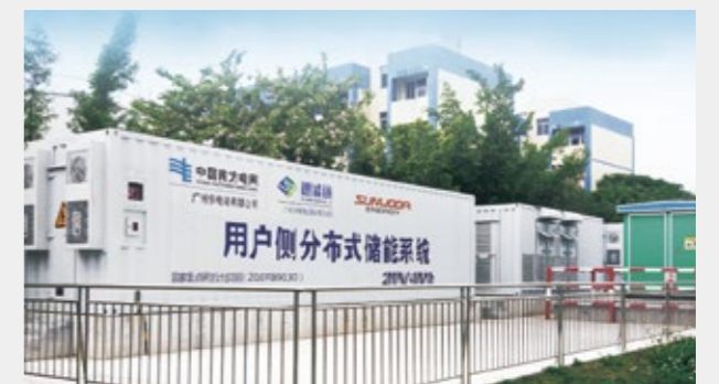
2MW/4MWh Guangzhou Industrial Park, Guangdong Province
