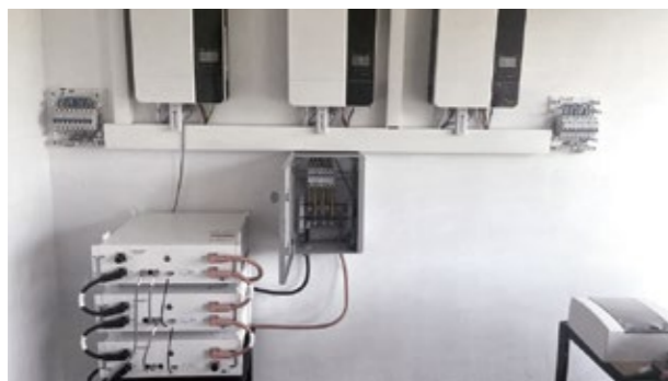
10kWh Bulgaria Residential Energy Storage Project
