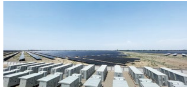
60MW/120MWh Jinta Photovoltaic Energy Storage System Project, Gansu Province
