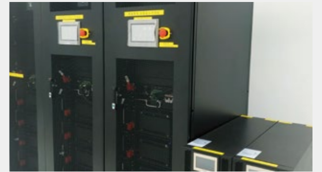
512V50Ah Backup Utility Project for Data Centers in Shanghai
