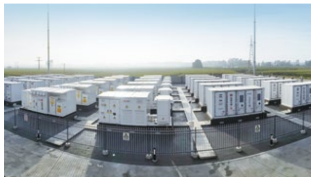
30MW/60MWh Neihuang Wind Utility Energy Storage System Project, Henan Province
