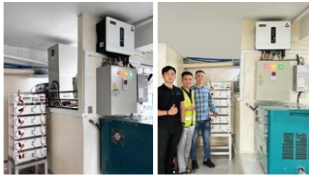
25kWh Vietnam Residential Energy Storage Project
