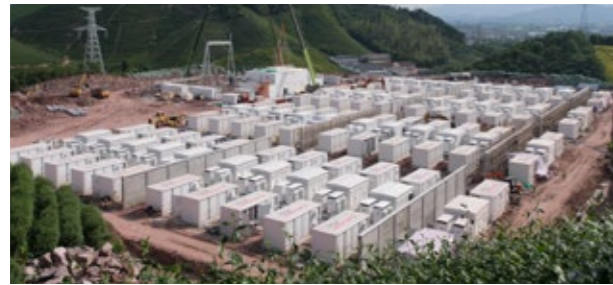
200MW/400MWh Grid-side Energy Storage Project, Zhejiang Province
