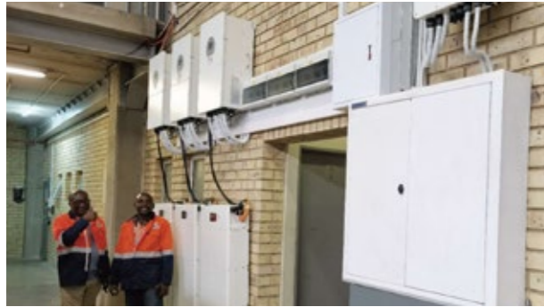
60kWh South Africa Residential Photovoltaic Energy Storage Project
