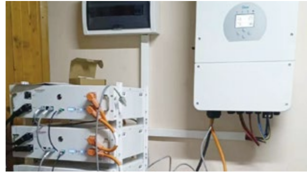
40kWh Greece Residential Energy Storage Project
