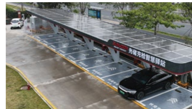
Shenzhen Photovoltaic-Storage-Charging-Inspection Project
