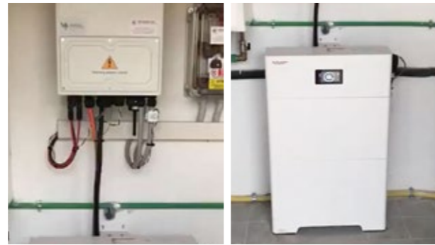
10kWh Italy Residential Energy Storage Project
