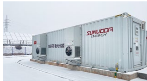
30MW/30MWh Datong Photovoltaic Energy Storage System Project, Shanxi Province
