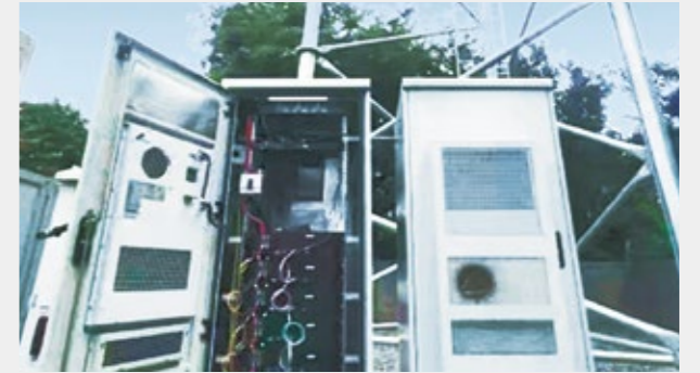
48V100Ah Backup Utility Project for Communication Base Stations in the Philippines
