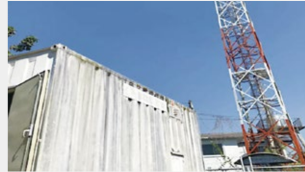
48V200Ah Collaborative Project with a Well-Known Telecommunications Company in Africa
