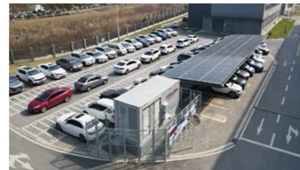
Nanjing Solar-Energy Storage Charging Project
