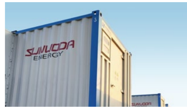
12MW/24MWh Xinhe Agricultural-Photovoltaic Complementary Energy Storage Project, Hebei Province
