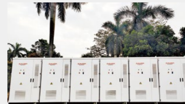
0.6MW/1.29MWh Huizhou Industrial Park, Guangdong Province
