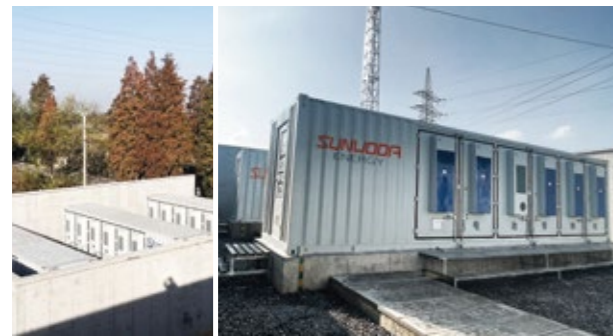
65MW/65MWh Qingyuan Agricultural-Photovoltaic Complementary Energy Storage Project, Guangdong Province
