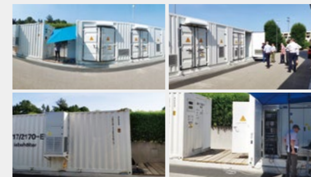
2MW/2.17MWh Switzerland Frequency Regulation Energy Storage Project
