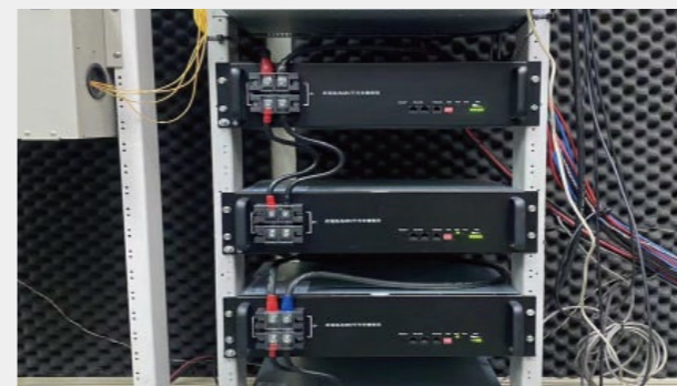
48V50Ah Backup Utility Project for Communication Base Stations in Taiwan, China
