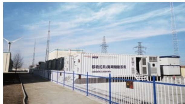
10MW/10MWh Shuozhou Peak Shifting and Frequency Modulation Demonstration Project, Shanxi Province
